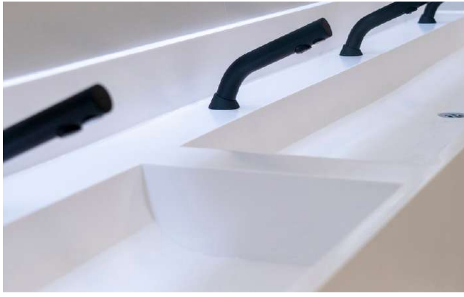
Can accomodate up to 5 users at once
