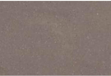
WX Weathered Concrete
