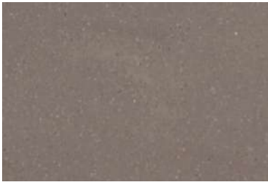
WX Weathered Concrete
