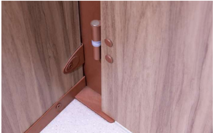
Bolt through brackets and hinges
